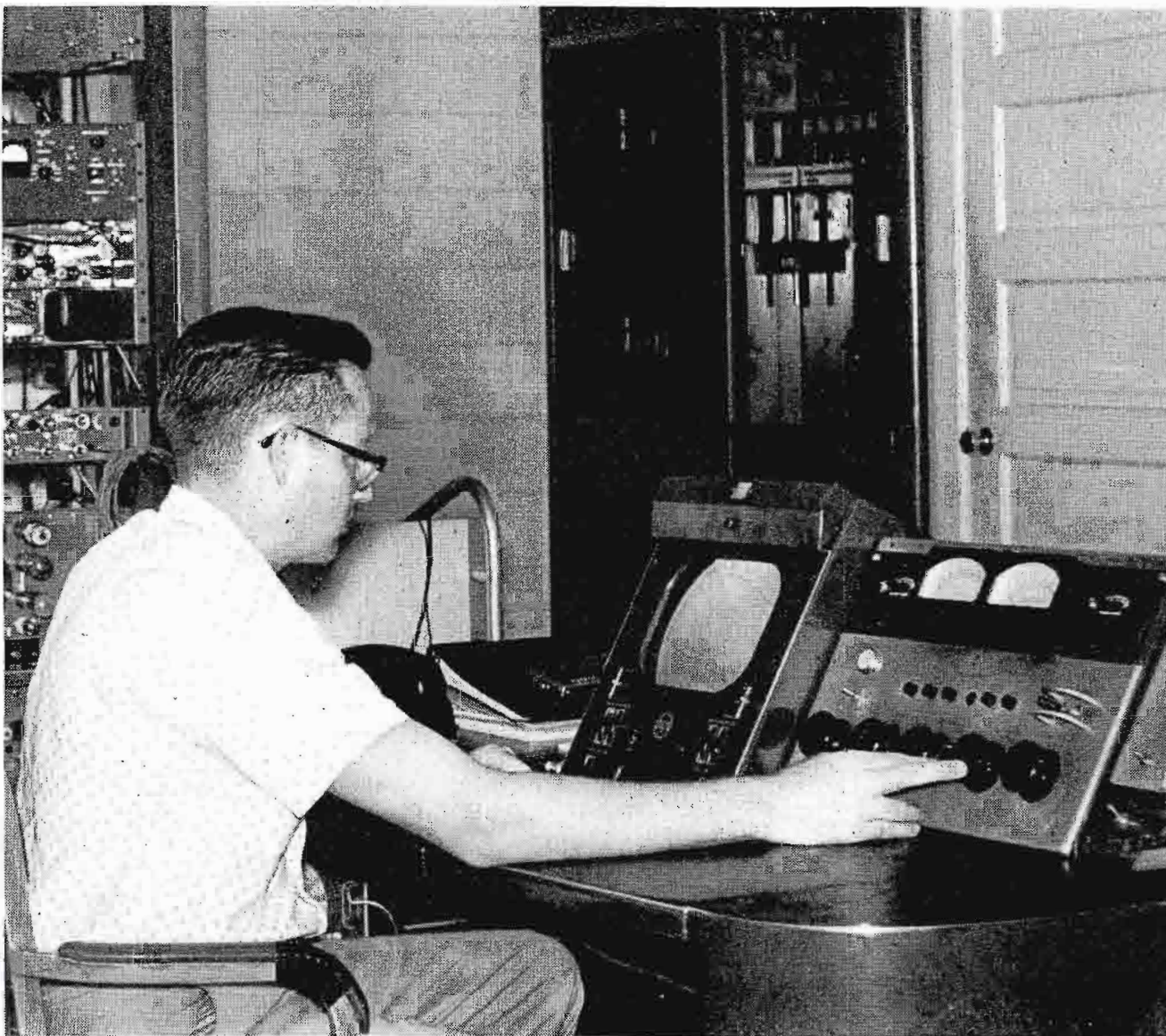
FIG. 12. WTVM transmitter plant. In foreground is the TTC-5 Control Console. At far background are the rectifier and control cabinets for the TT-25CH aural power amplifier.
